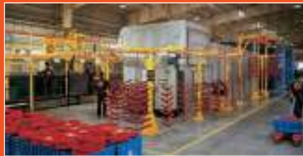
Robotically armed & conveyORIZED double booth powder coating plant with a capacity of 15 million sq inches / month
